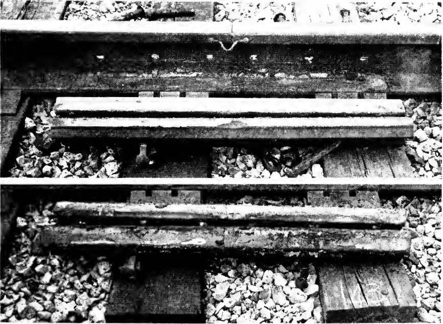
Fig. 22. 131 RE H. C. Rail Joint with Brush Coat of Petrolatum (Dark) After 4-years' Service in the Westward Main of the Burlington Railroad near Earlville, Ill.
